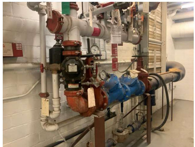
24 - FIRE SUPPRESSION SYSTEM
